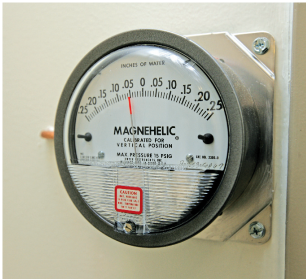
FIGURE 16. Magnehelic Gauge for Visual Confirmation of Pressurization
