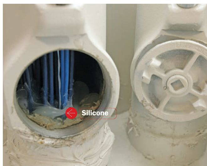
FIGURE 1. Caulking around Service Intrusion*
